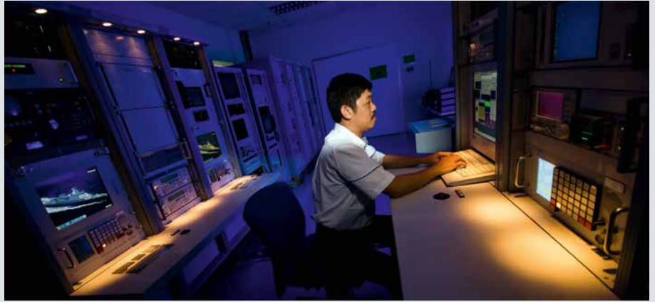
An integrated communications system from Rohde & Schwarz is installed aboard this Royal Malaysian Navy (RMN) Kedah class patrol vessel.
